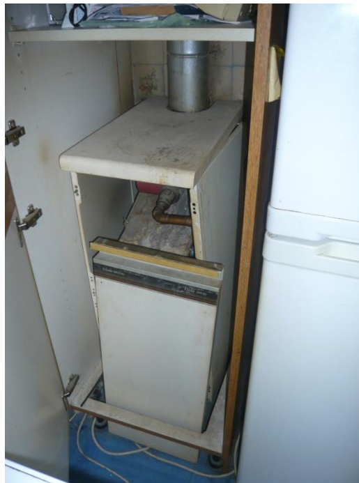
Figure 6 - Boiler in household 3 (Sally)
